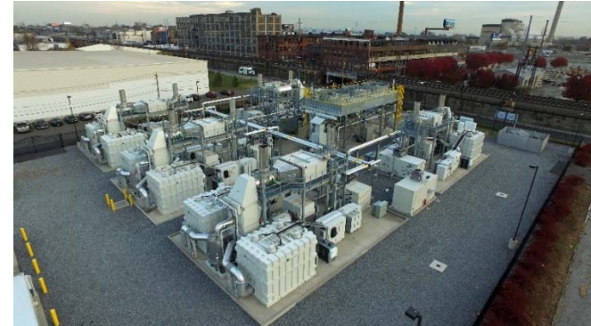
14.9 MW Bridgeport, Ct (FuelCell Energy)
